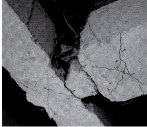
Figure E2-23 Database joint J5 (Specimen RE1) during repairs, following removal of loose concrete. Photograph obtained from Tsonos and Papanikolaou (2003).
