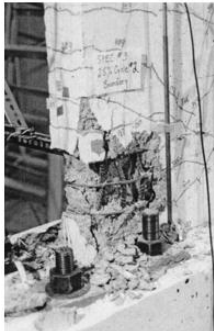
Bar buckling and concrete crushing (Thomsen and Wallace, 1995)
